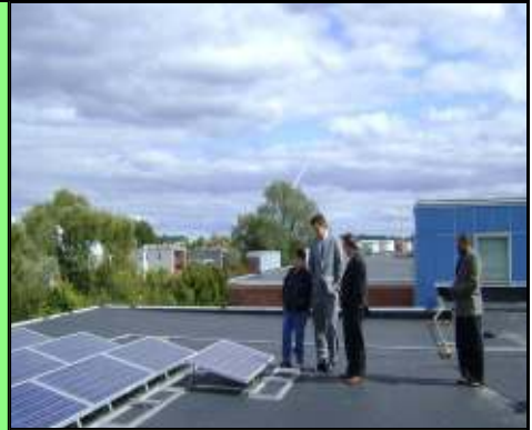
The City's first solar panel installation took place this past year at the Burke School Complex on Eastern Avenue.
