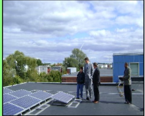
The City's first solar panel installation took place this past year at the Burke School Complex on Eastern Avenue.
